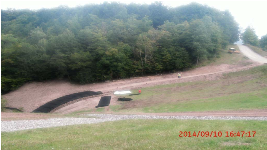
Placing Topsoil on the Lake 2 Overflow Plume and Installation of Enkamat Matting
