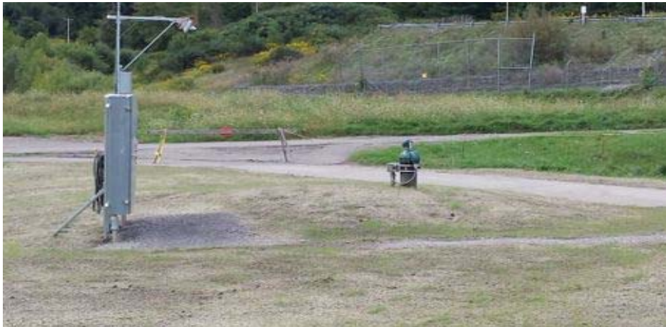
Completed Well 1 Showing Electrical and Wireless Panel
